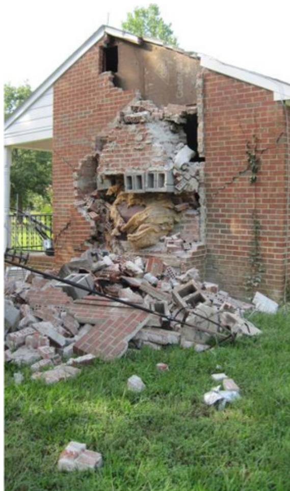
Chimney Damage in Louisa County (epicenter)
